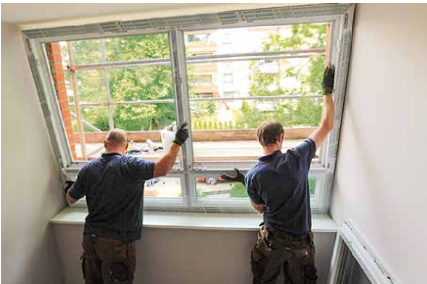
The perfect fit, just in time – the installers fit the new windows as soon as they are delivered.
