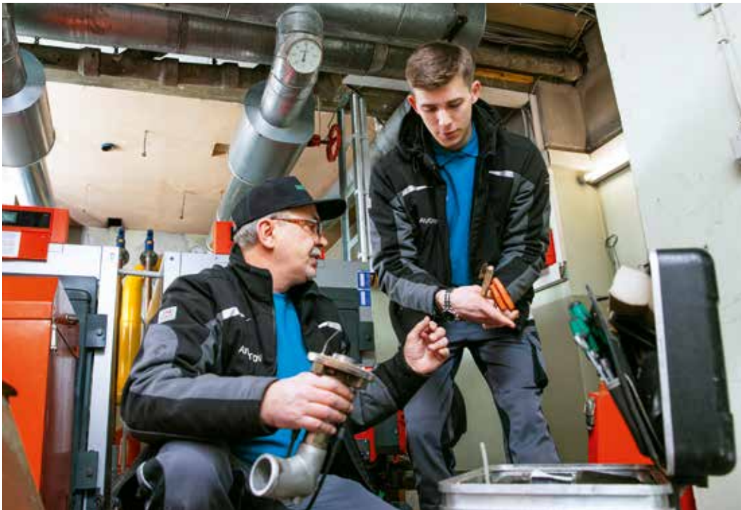
Practice makes perfect: Ulrich Hagemeyer, a heating and air conditioning engineer for Vonovia's technical service, and trainee Vyaceslav Goncharov at work.
